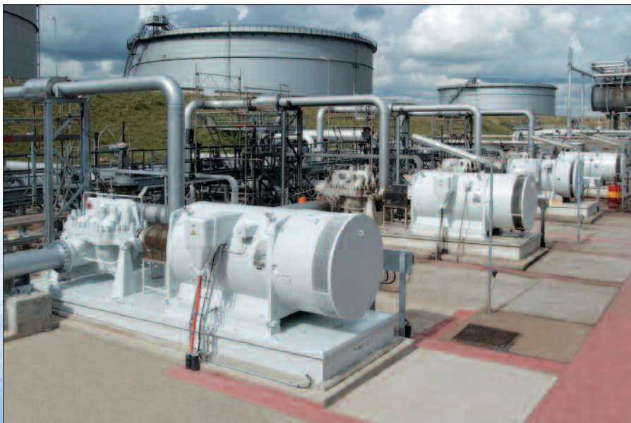
Drives for crude oil pumps, Exd(e) IIB T4, 1,500 kW, 10 kV, 4pole
