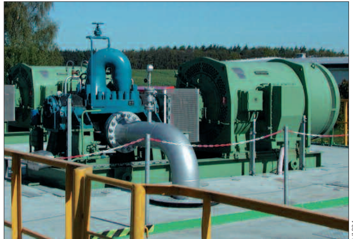
Pump drives in a pipeline booster station, Exd(e) IIB T4, 1,450 kW, 6 kV, 2pole
